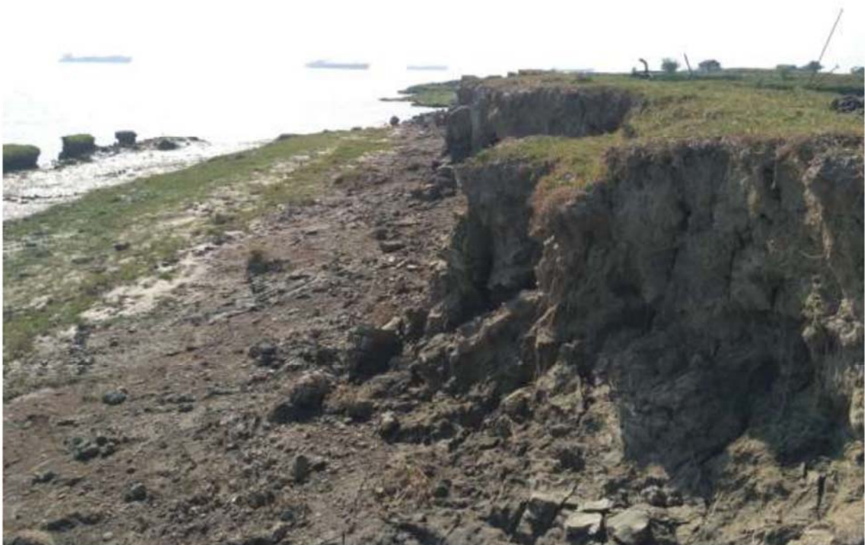
Plate 144 – Bank Erosion , Haldi River , Haldia 22° 1'1.93"N 88° 3'30.71"E
